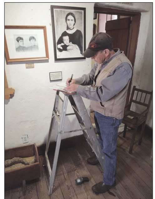
Roy Woods of Conron & Woods inspects the interior walls of the Carson House.
